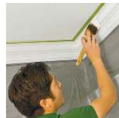
Cover walls and ceiling with tape. Using brush, coat cornice with paint.
