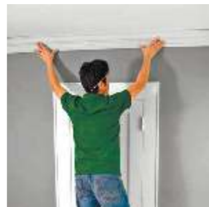
Make markings on the wall using a pencil to define the cornice location
